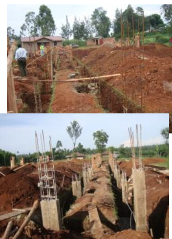
Two early dormitory construction scenes: top, preparing the footings to support the upper floor and roof (see the Administration Block in the distance); bottom, the support columns begin to
